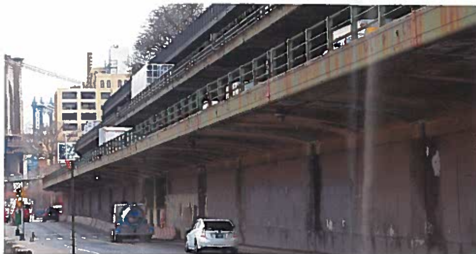
The BQE consists of 21 bridges including a unique triple cantilever structure. This portion of the highway carries a daily traffic volume of 140,000 vehicles.
